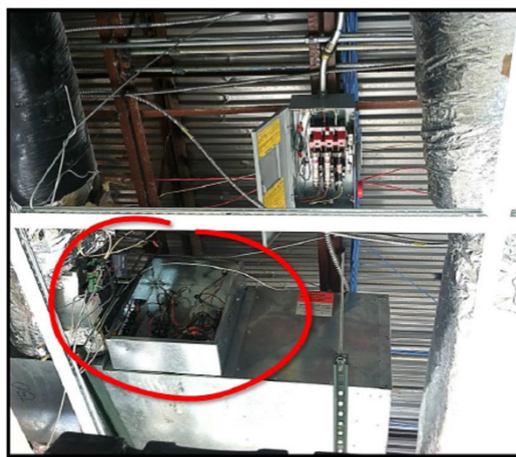
Working space is required above the ceiling at duct heaters.
