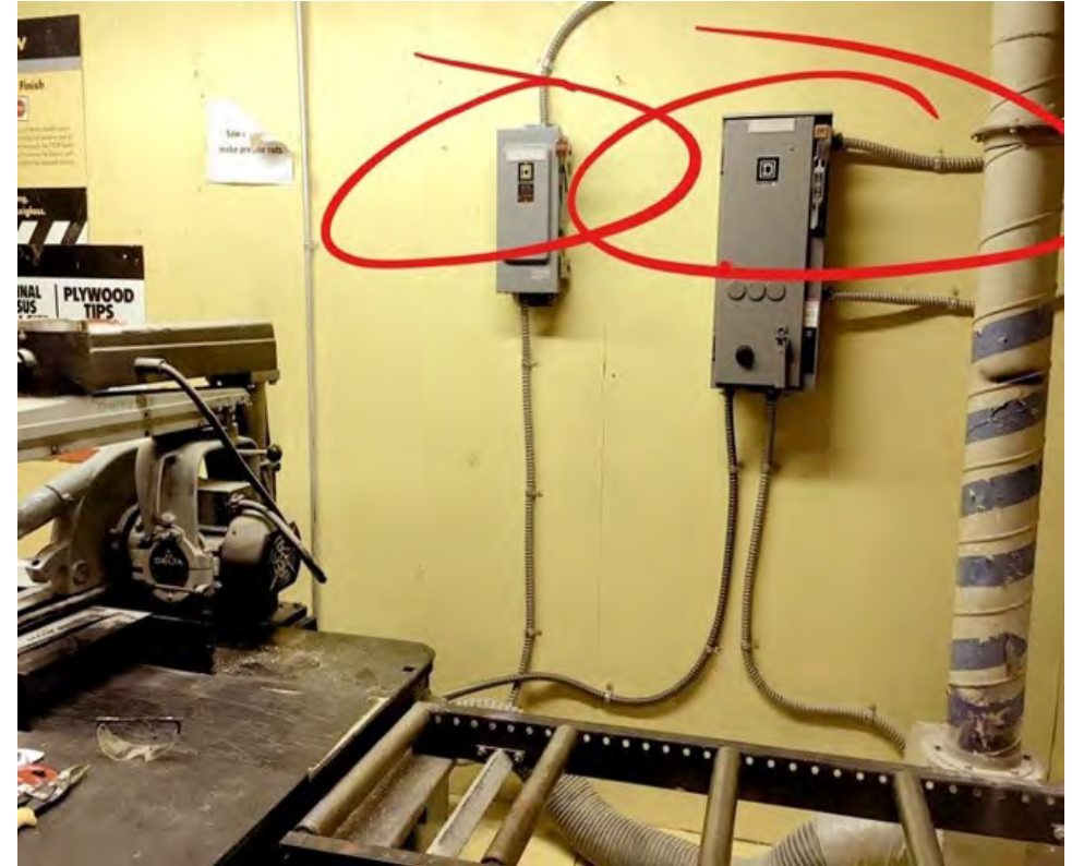
Two energy isolation devices (disconnects)
