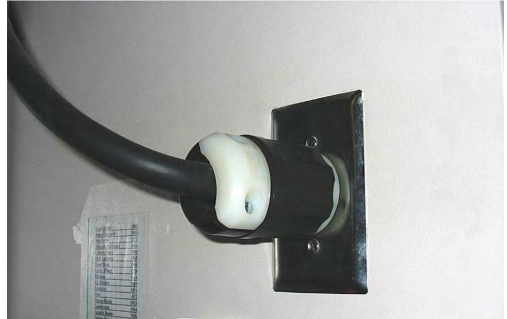
Stationary cord-and-plug connected equipment
