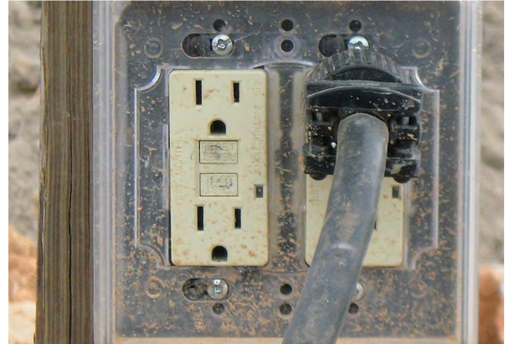
Outdoor GFCI Protection
