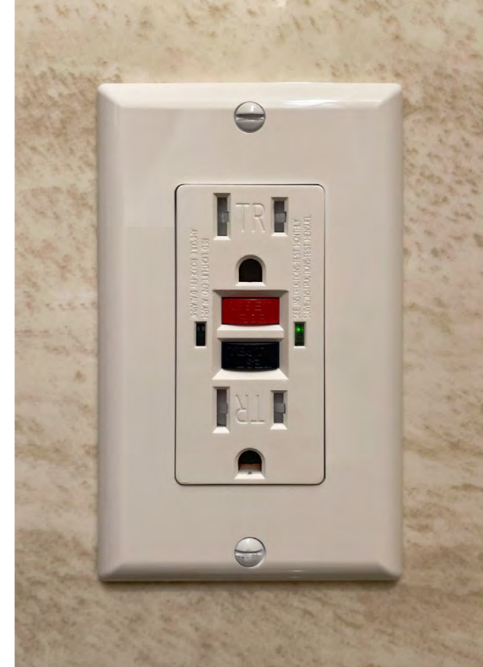
GFCI receptacle with red button for Reset and black button for Test
